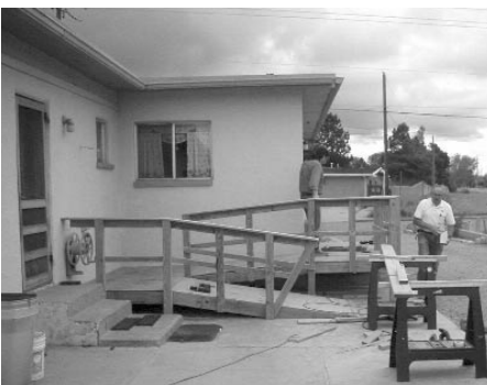
Charles Lury constructing a home-accessibility ramp for a disabled client, one of the 170 individuals able to continue living in their homes last year thanks to necessary modifications by OPEN HANDS staff.
