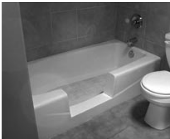
New TubcuT™ installation increases access and safety for seniors and their caregivers.
