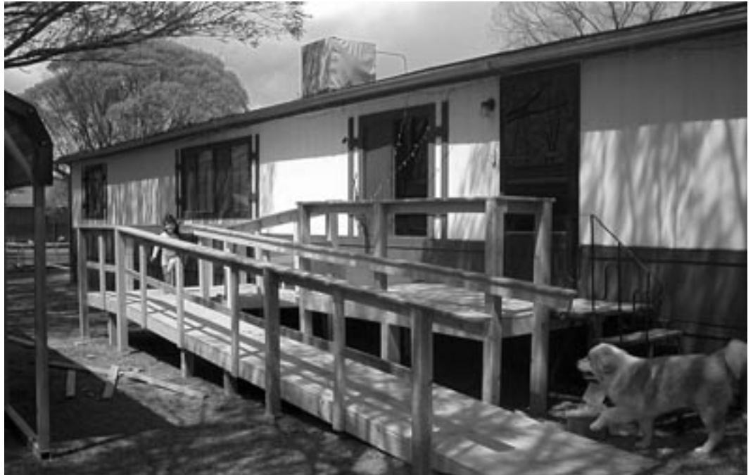
A wheelchair-accessible ramp crafted by COS Home Safety installers for a local area home.
